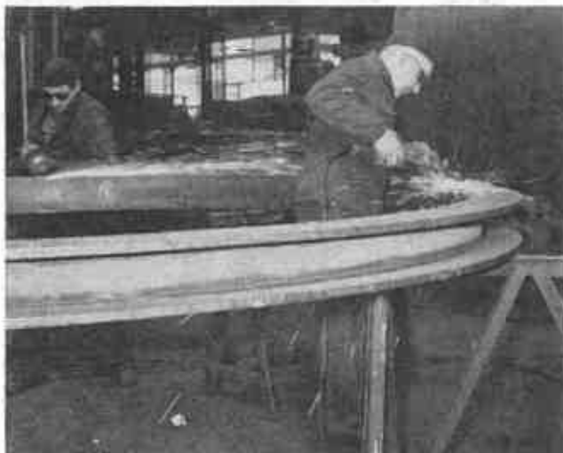
Fig. 3—Grinding one of the 16 stiffener rings used to reinforce the 33-mm-thick hull shell.
